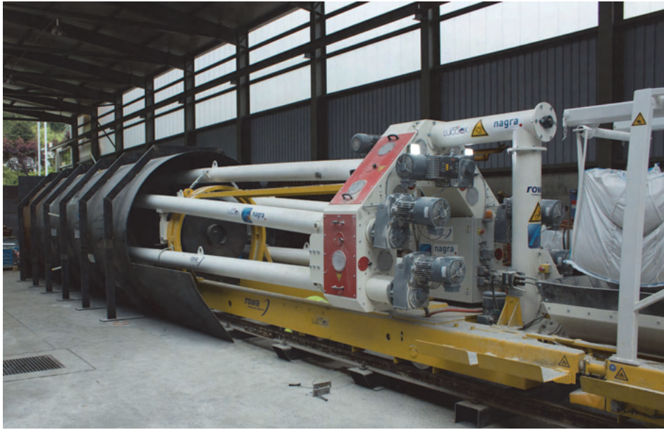
Fig. 2.3: Multiple-screw-conveyor machine used to emplace the bentonite backfill material in the triple-heater repository scale test at the Mont Terri rock laboratory. Here the machine is used in a mock-up pre-test. Note the dummy canister between the conveyor pipes at left.
