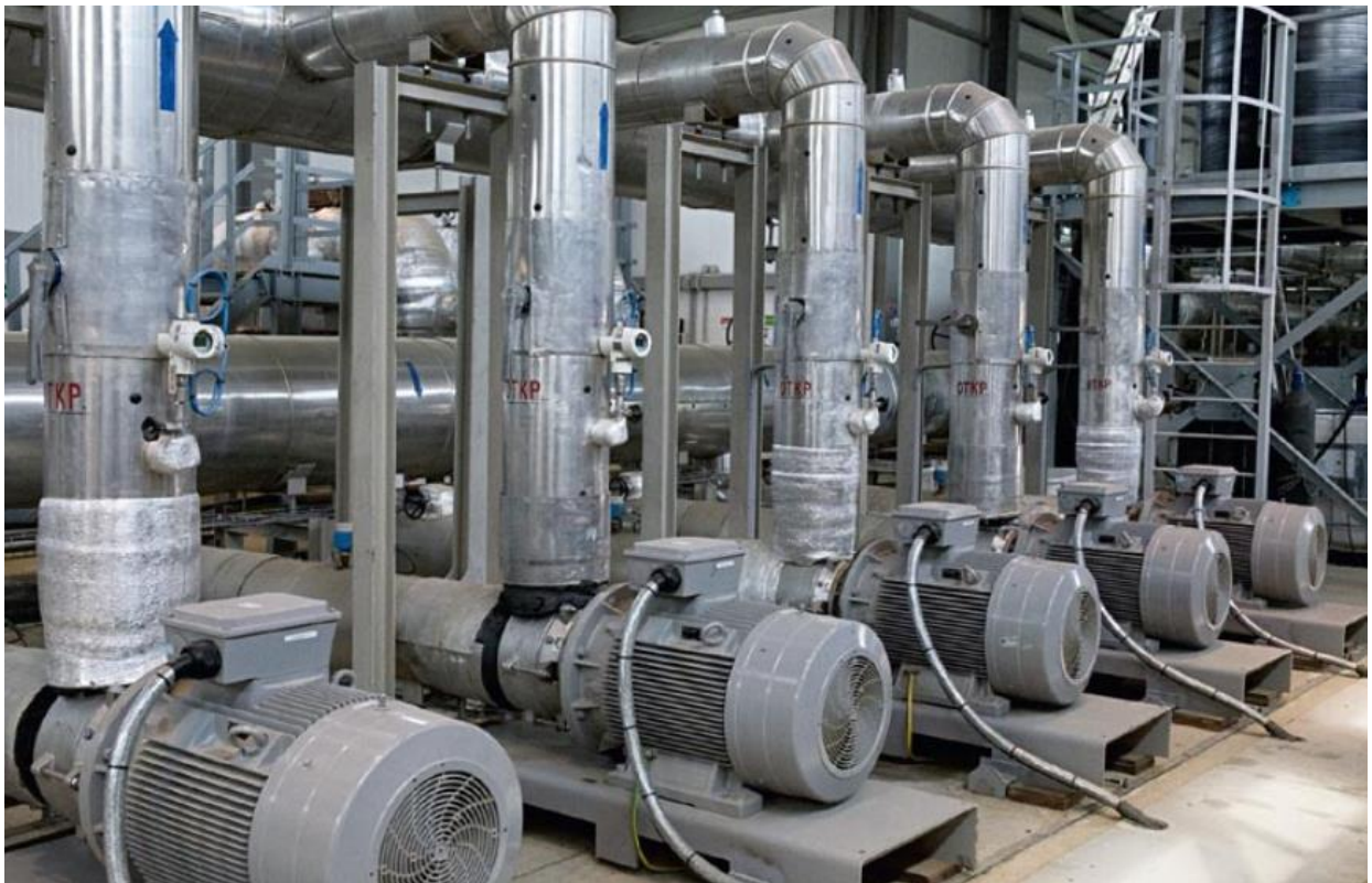
Fig. 2: Freezing plant at a Potsah mine and corresponding brine pumps (Van Heyden & Wegner, 2015)
