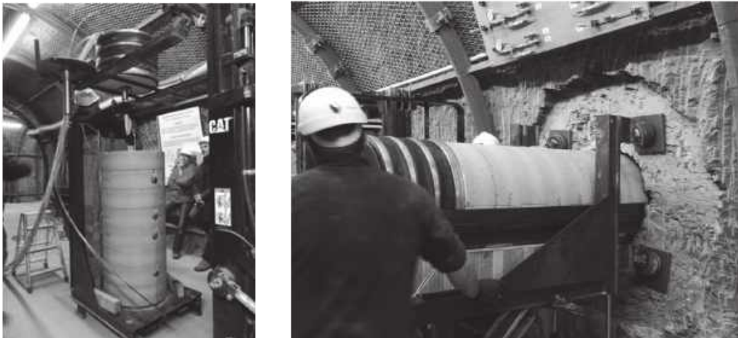
Fig. 1.1: Preparation of the plug from eight BSM blocks and its horizontal installation.
