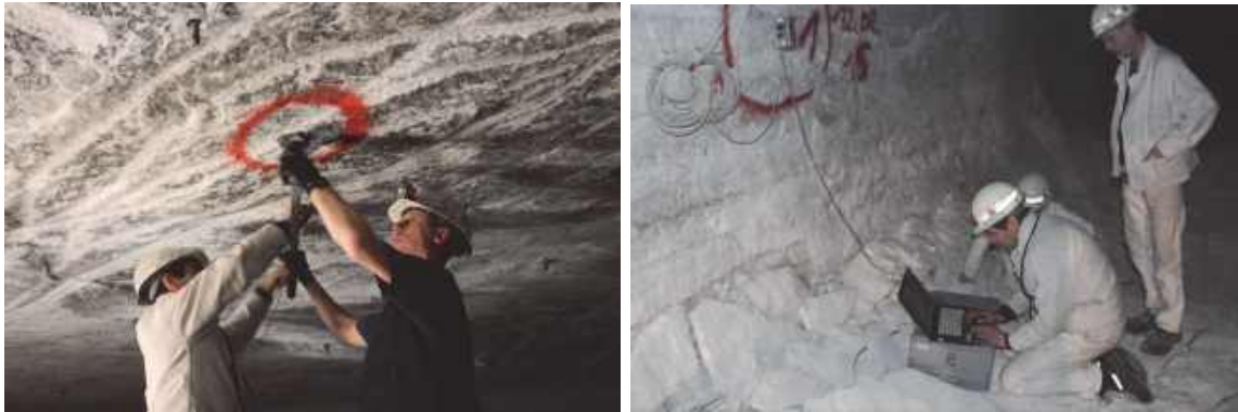
Fig. 4.2: Working activities during the installation of the measurement device. Left picture: Pre-tensioning of the custom-made bolts using a torque wrench. Right picture: Setup of the data processing and logging unit.
