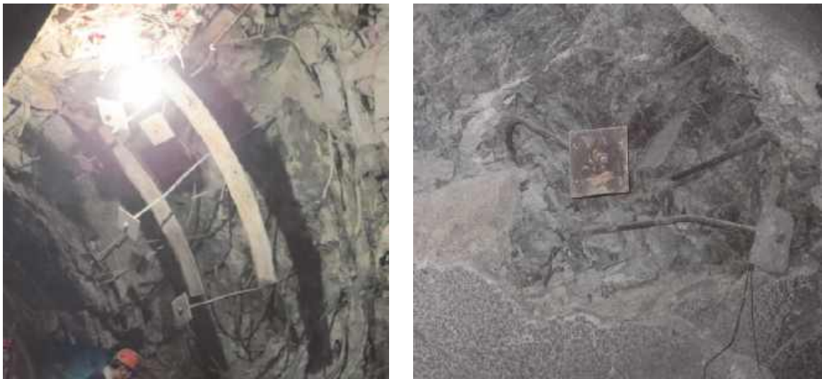
Fig. 6 The failure characteristics of bolt in original support
