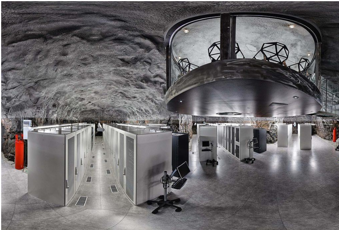
Fig. 7.1: Data centre and office building of the Swedish internet-providing company Bahnhof AB (UGE, 2020)
