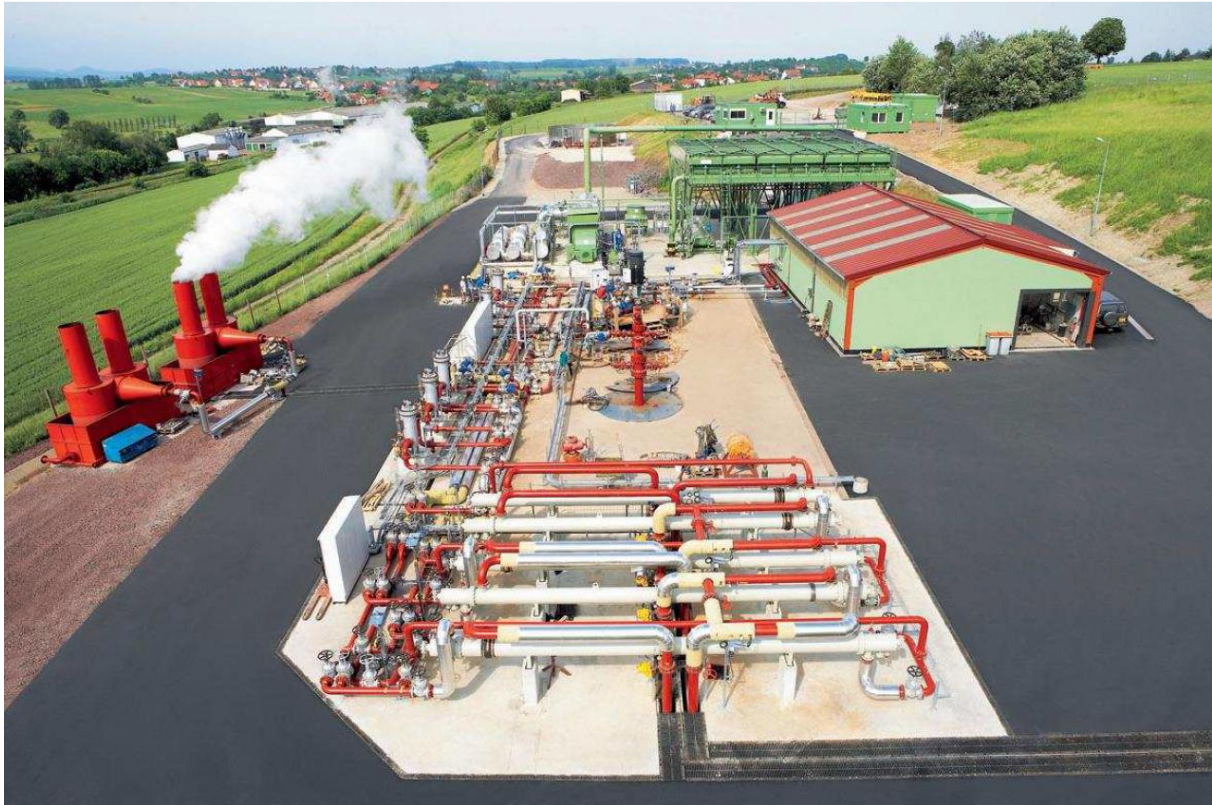
Fig. 5.2: The geothermal power plant EGS Soutz (Genter et al., 2009)
