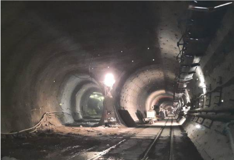
Fig. 3.5: Intersection of northern tube (TBM) and access tunnel north (courtesy of Geoconsult ZT GmbH).
