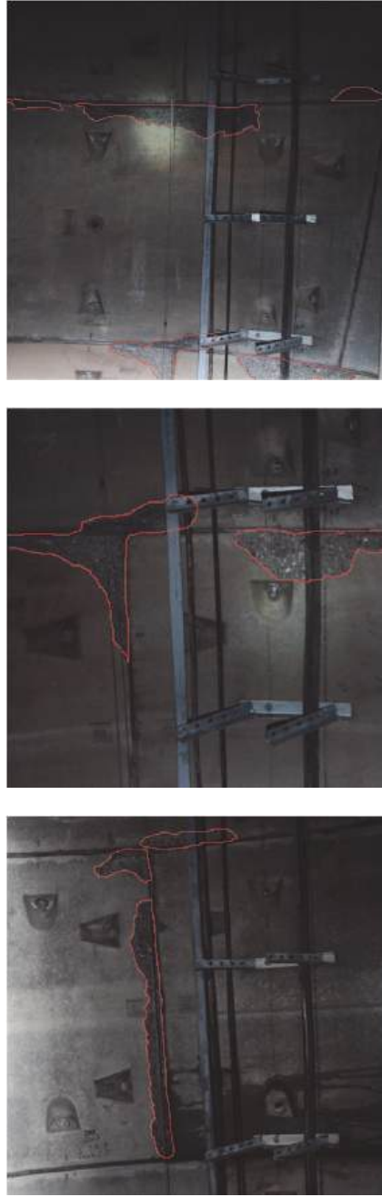
Fig. 17: Large-scale irregular spalling caused by the construction of a foundation pit
