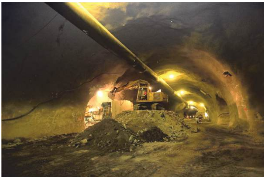
Fig. 3.1: Emergency stop – logistic cavern (courtesy of OeBB).
