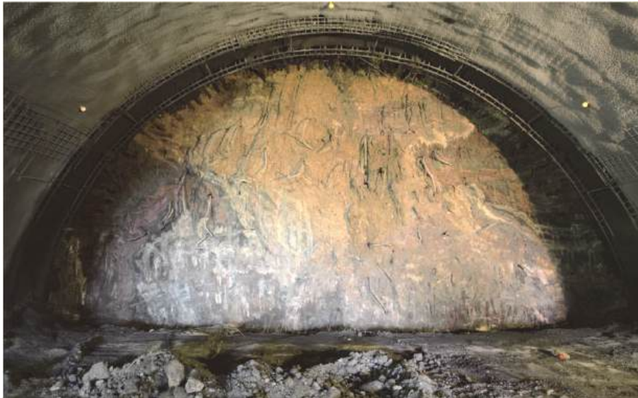
Fig. 3.2: Top heading face showing mixed face conditions with competent rock alternating with soft ground.
