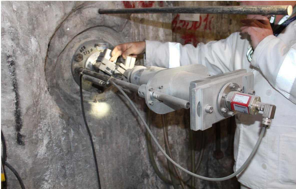
Fig. 4.1.5. Extensometer head (installation in an underground mine)
